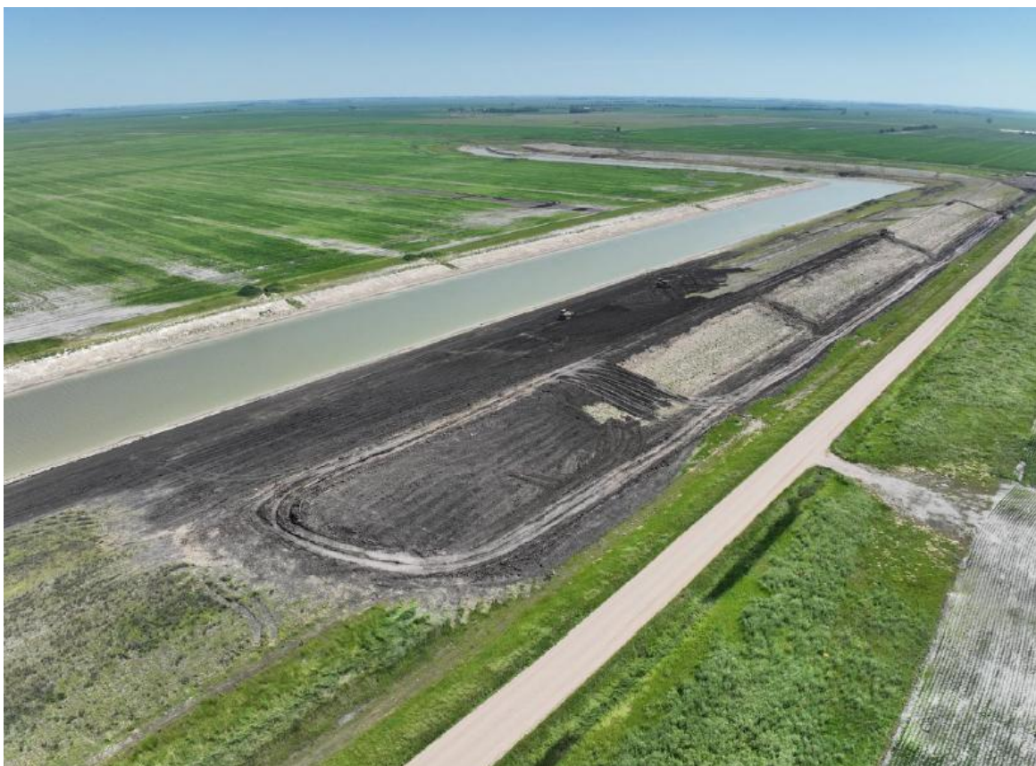
John Riley Construction pulled material from inside of the Redpath Flood Impoundment to build the Impoundment walls.
